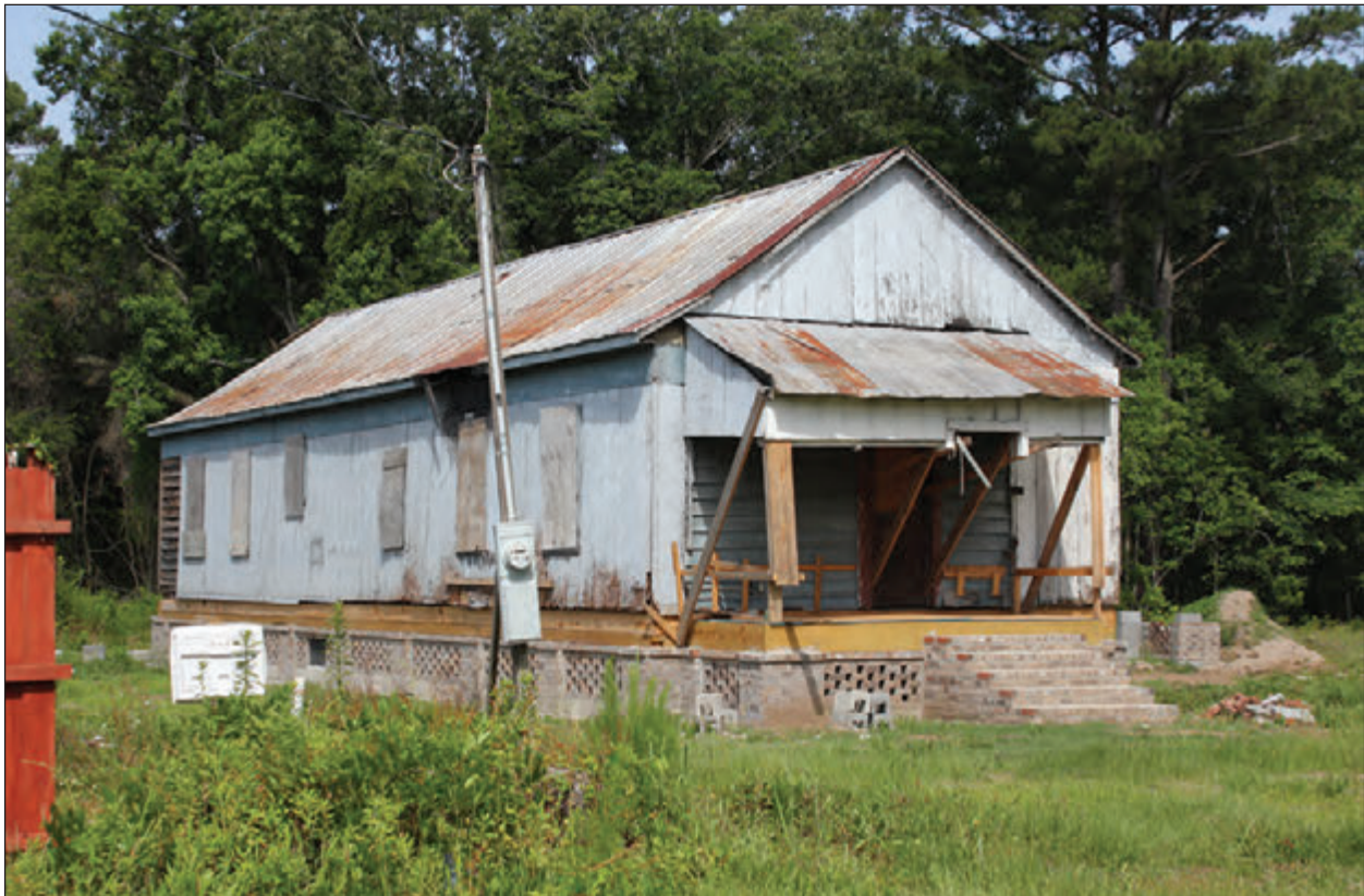
Figure 6.3 Long Point School (SHPO Site No. 7802), at original location in 2018, facing northwest (top), and at its current location, facing southeast (bottom).
