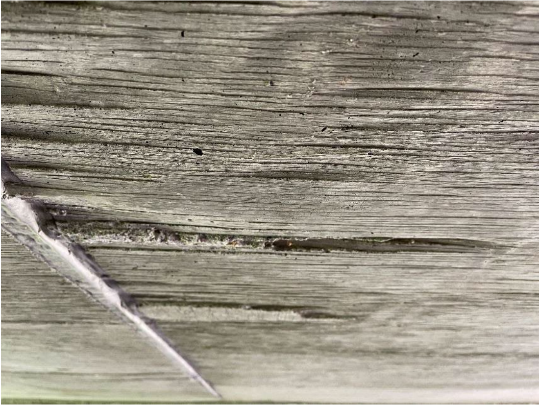
Photograph 11: Rough surfaces under the decks of tidal creek bridges
